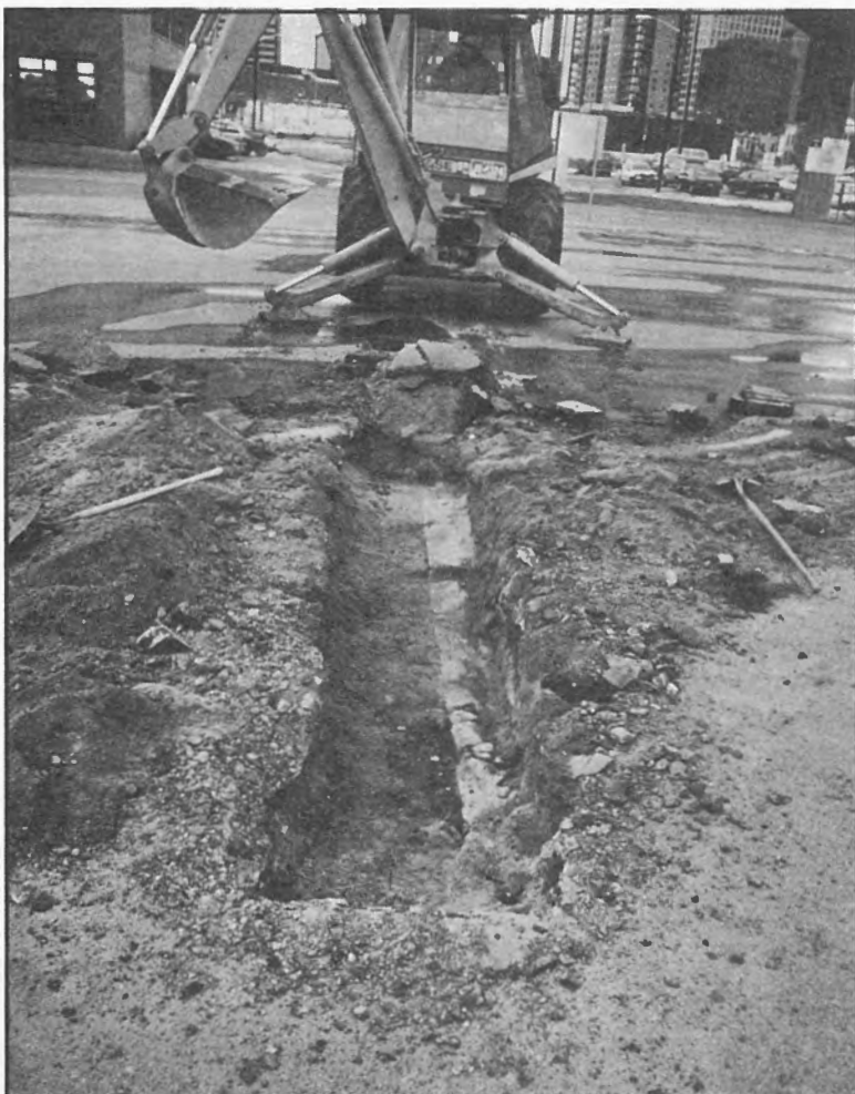
Figure 9 - A brick foundation wall beneath the asphalt surface exposed during test excavations.
