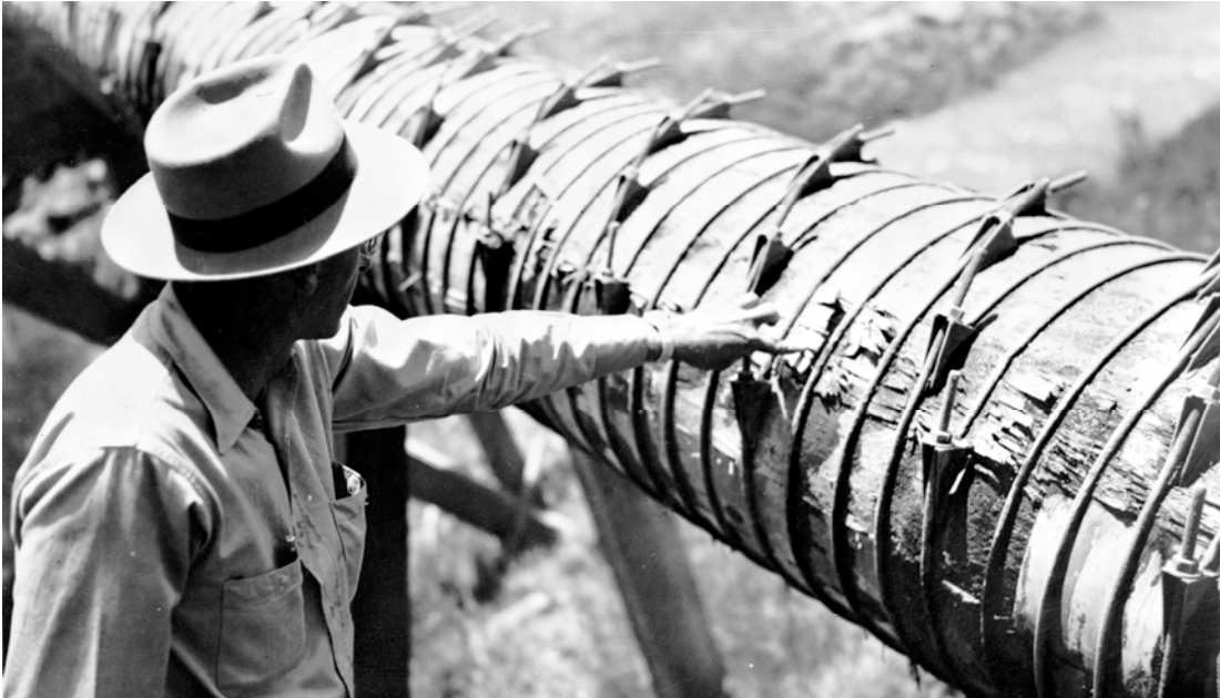
Figure 19. Wood-stave siphon pipe on the Montezuma Valley irrigation system, constructed c. 1885, photographed in 1951.
