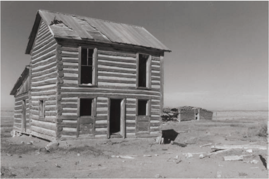
FIGURE 5. Photograph taken in 2002 of the Pedro Trujillo log house (Feature 1), view northwest. The stable/barn (Feature 2) is visible in the right background.
